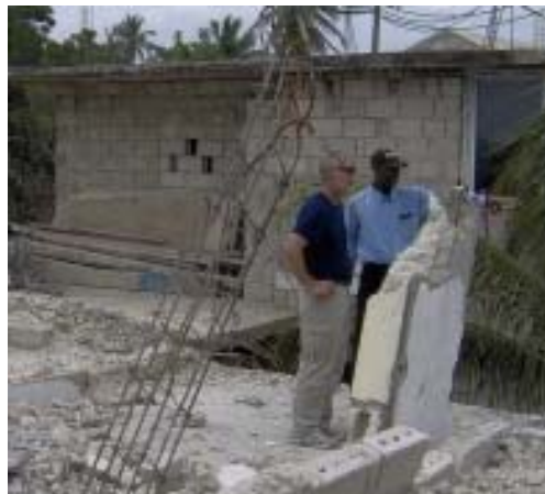
David and Yvon survey damage at Santo School
