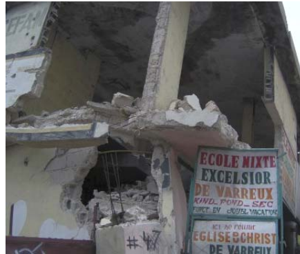
Earthquake damage at Varreux
